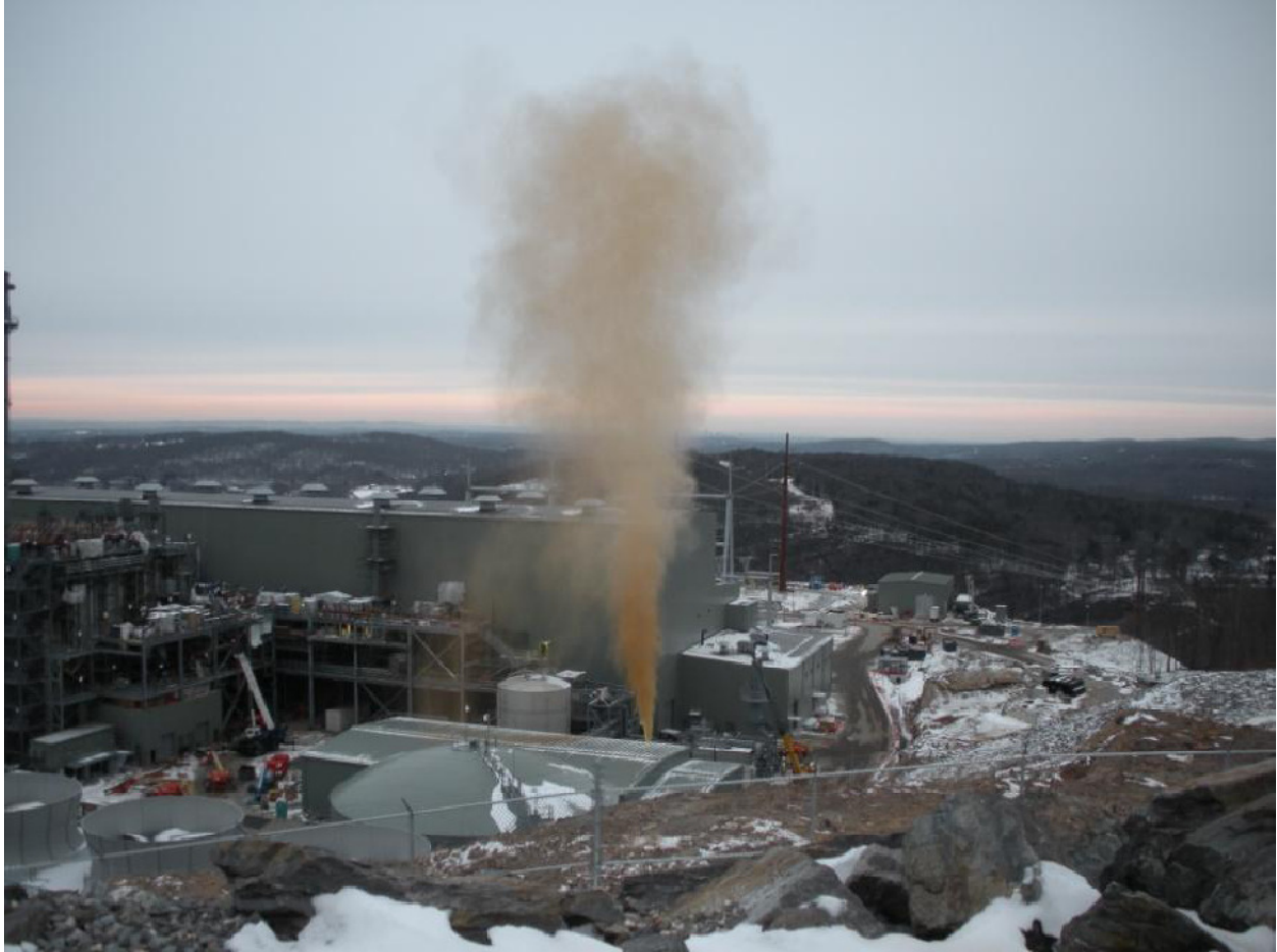
Figure 4. A gas blow from an electric power plant used to remove debris from piping. The brown cloud represents debris in the lines. Photo, Kleen Energy, 30 January 2010, as used in a CSB report urging changes in regulations and standards, http://76.227.217.14/UserFiles/file/FINAL%20Urgent%20Recommendation.pdf .
