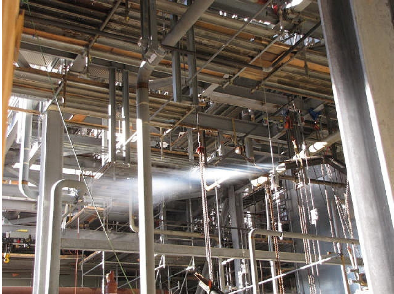
Figure 1: Natural gas venting during purging of lines, photo taken on Feb. 7 before explosion (used in CSB report)
